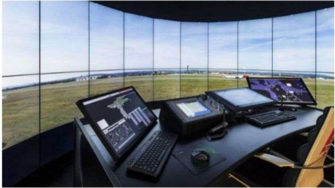
Control system at an airport
