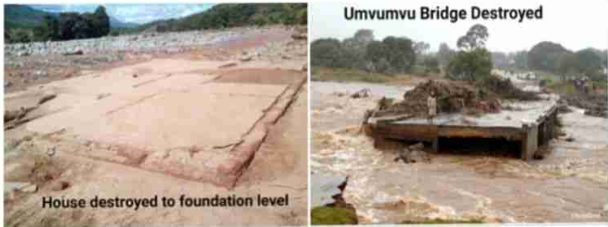
Fig 1.8: Cyclone Idai damaged infrastructure and homes Source: Stanely Duri (2019)
