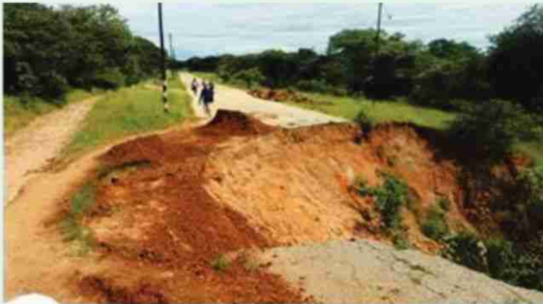
Fig 8.2: Soil Erosion in Gokwe destroying the road
