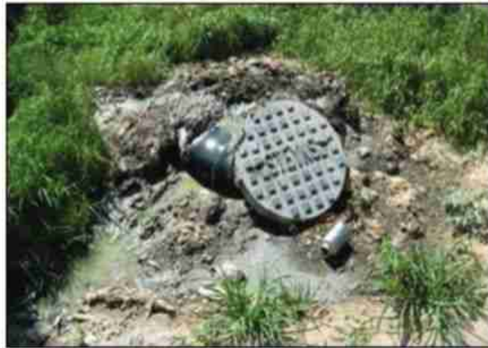
Fig 11.2: Burst sewage pipes
