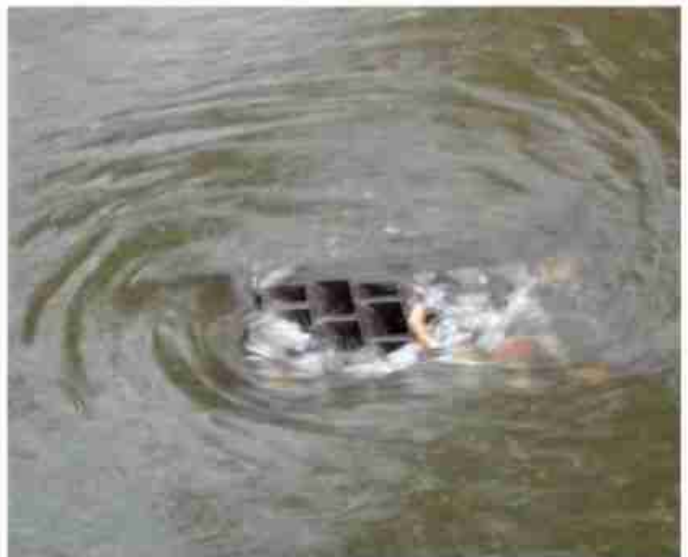
Fig 1.3: Blocked drainage pipes increase the risk of flooding
