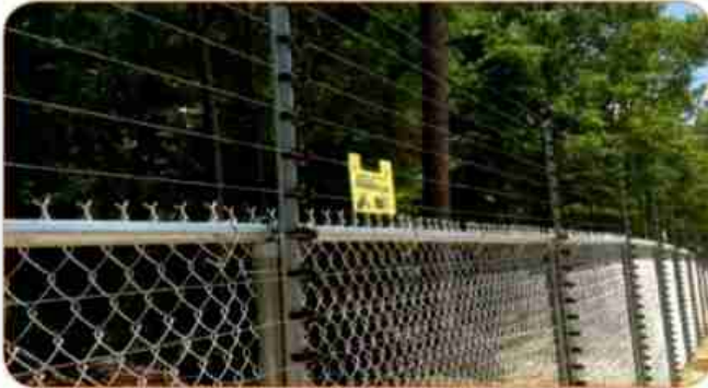
Fig. 9.13 Typical electric wire fence
